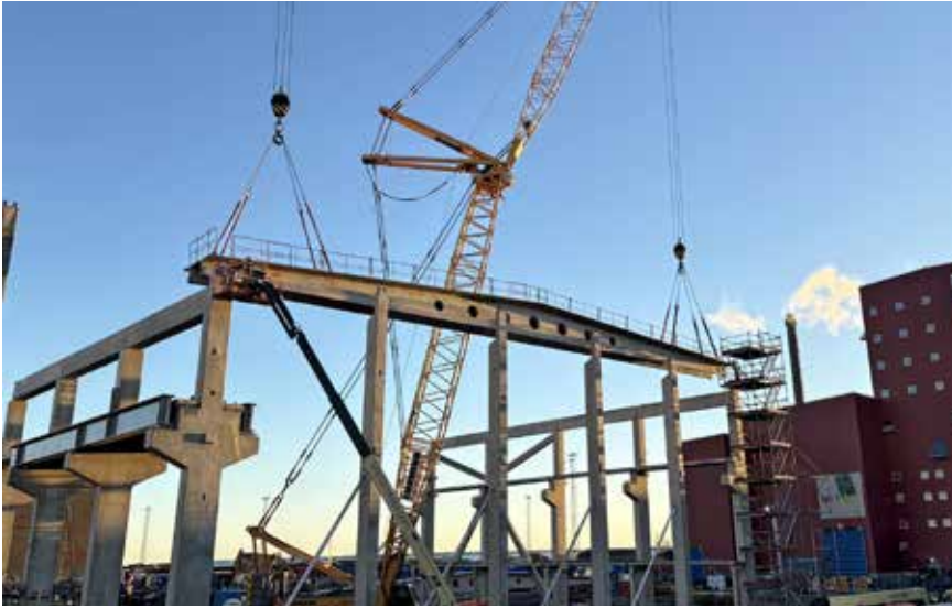
Roof truss prepared with integrated sprinkler systems, installed at ground level before being lifted into place
